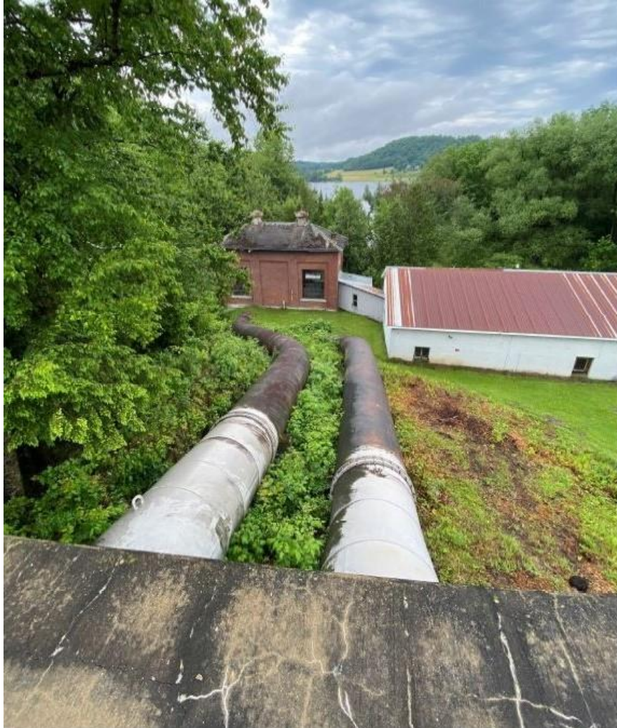
Photo of the penstocks at Barton Electric's Hydroelectric Facility
